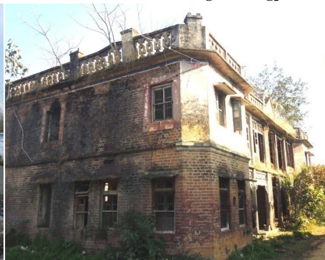
Poor Restoration of Buildings in Pragpur
